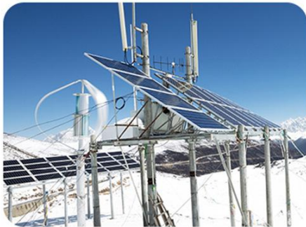
Mountain communication base station
